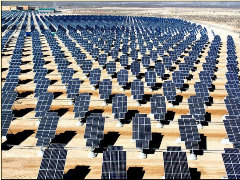
Solar voltaic power plant
