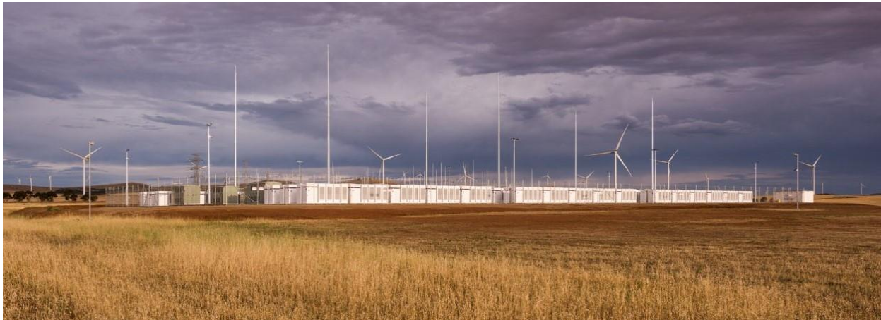
World’s largest lithium ion battery, surrounded by the Hornsdale Windfarm ( http://www.ecogeneration.com.au/worlds-largest-tesla-battery-switches-on-at-hornsdale-wind-farm-south-australia/ )
