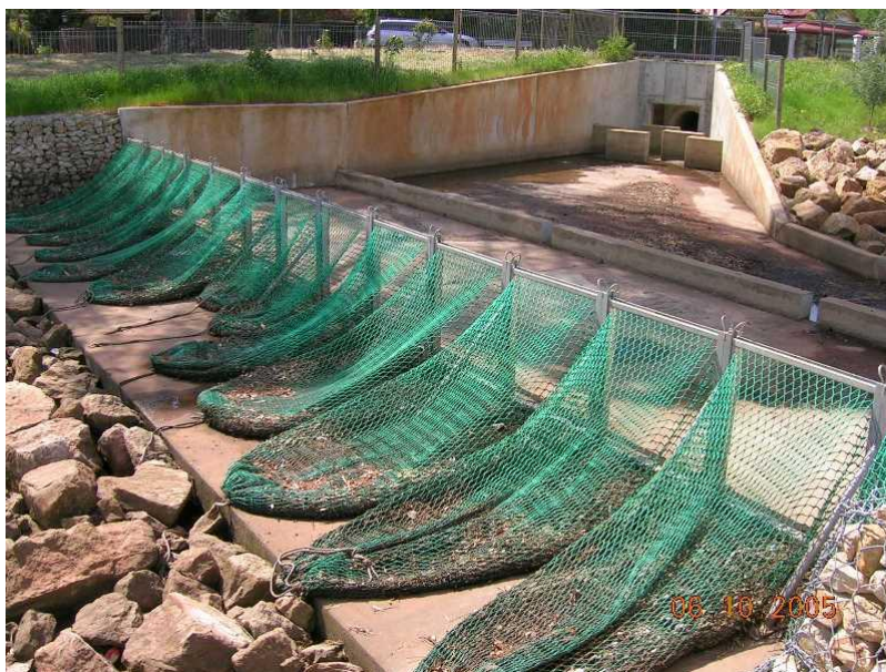
Trash racks capture rubbish transported in storm-water at the Urrbrae wetland in suburban Adelaide. http://www.mitchamcouncil.sa.gov.au/webdata/resources/images/DSCN2655.JPG
