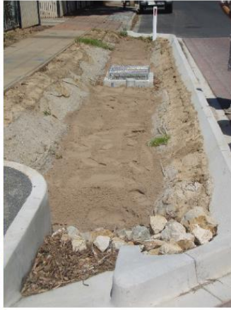
Rain garden bio-filtration system, prior to planting, City Of West Torrens
